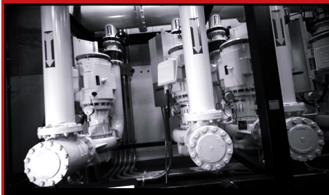
MOTORS, PUMPS, HVAC, PIPING AND STRUCTURES
